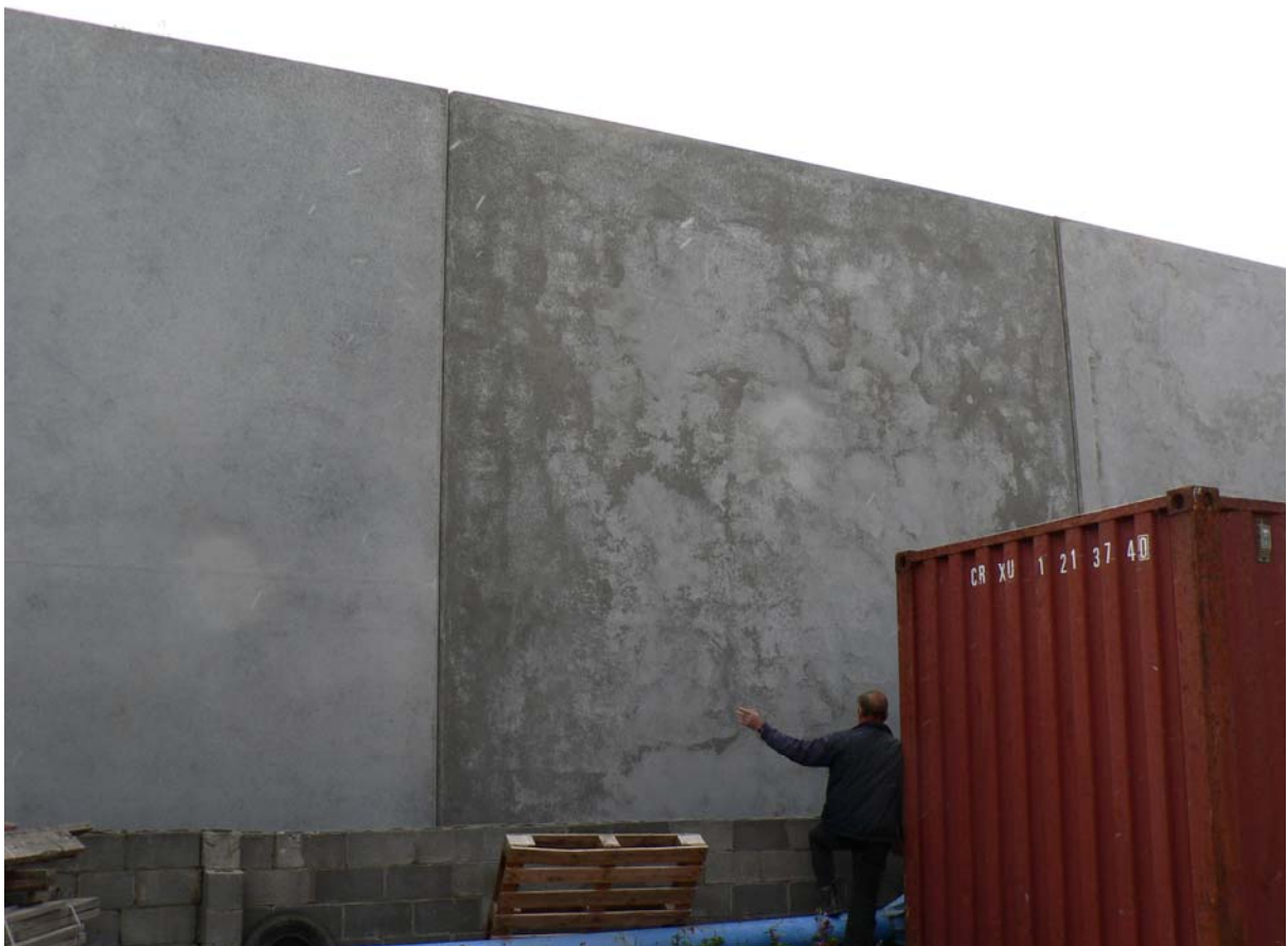
John Higgins Pointing out the Bleed Marks and Segregation on a non Tec-Cement Tilt-Up. Tec-Cement Tilt-Ups Either Side.
